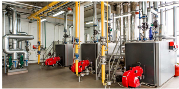
Energy Efficiency and Water Conservation Upgrades at Hilton Bayfront, San Diego, CA
