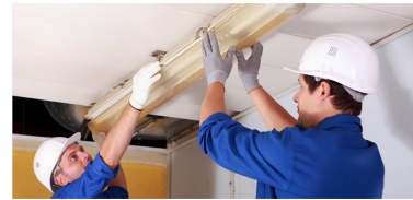
Direct Installation of Energy Conservation Measures (largest direct install program in the country), Con Edison Small Business Direct Install, New York, NY
